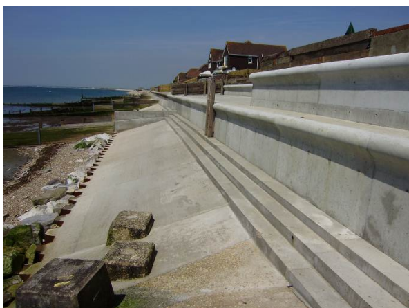
Photo 2.2: West Beach, Selsey. Beach levels prior to the 2011 Selsey West Beach Recharge scheme.
