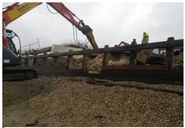
4. Breastwork failure at East Wittering as a result of undermining due to low beach levels 6 th January 2014
